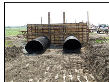
Pipes and concrete forms for one of the sediment containment outlet structures
